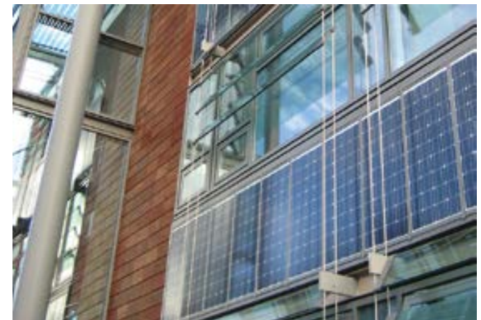
Integrating micro renewables—Kings Buildings Solar Panels are integrated into the design of the elevation.
