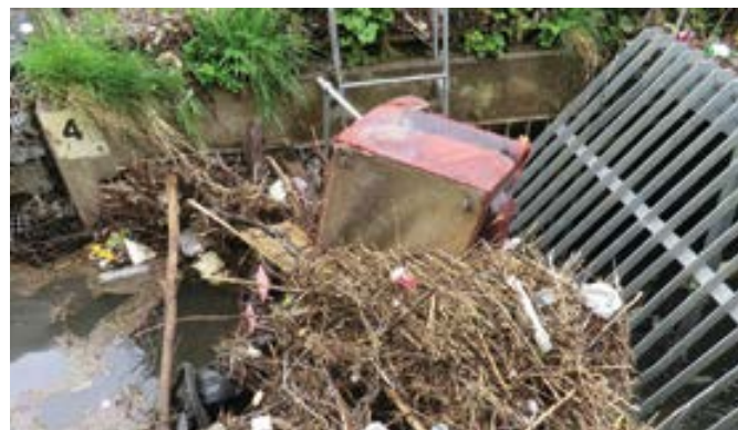
locked up culvert
