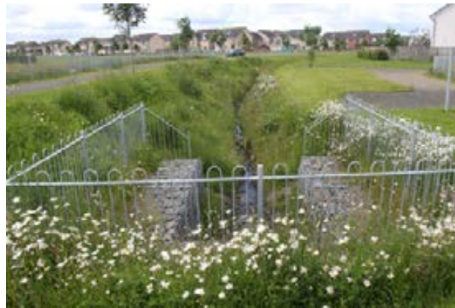
SuDS retention basin and swales, Kirkliston
